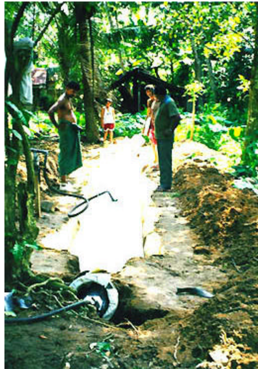
Fig 1. The biogas plant. Gampaha, Sri Lanka
