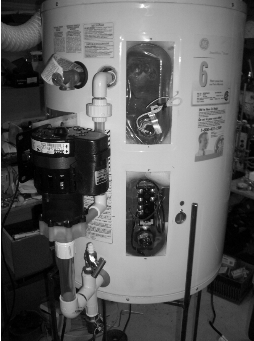
Photo #16 Recirc pump and Methoxide valve mounted. System ready for leak testing.
