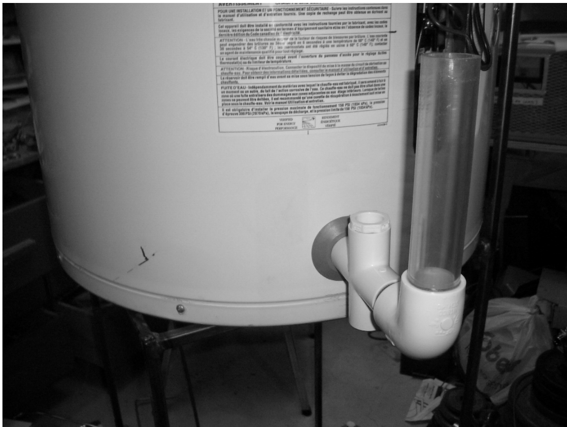
Photo #14 Building inlet manifold.
