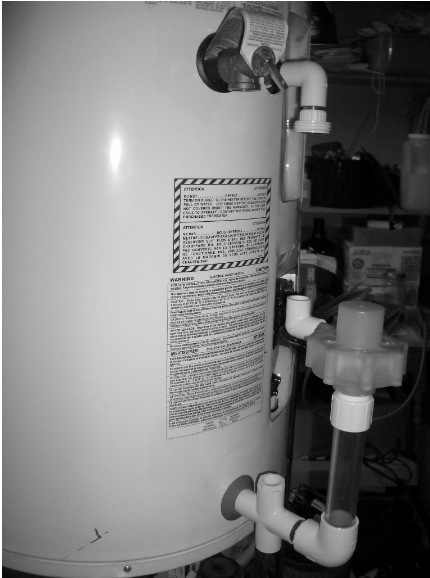
Photo #15 Building Recirculation loop.
